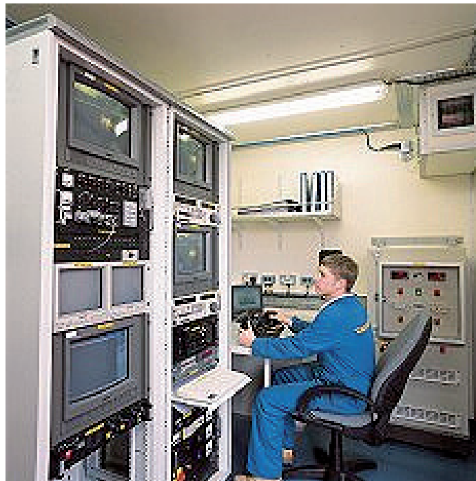
Figure 32: A typical control room. (Source: http://www.subfind.com/panther.htm )
